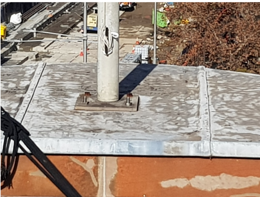
Figure 4: Corroded Flag Pole Connections South End
