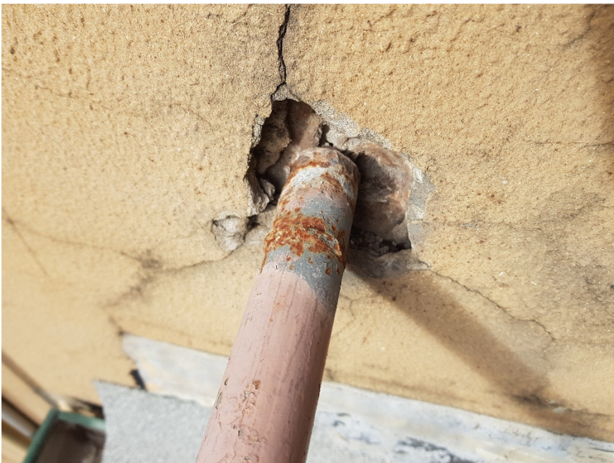
Figure 8: Original Railing Broken Off from Wall
