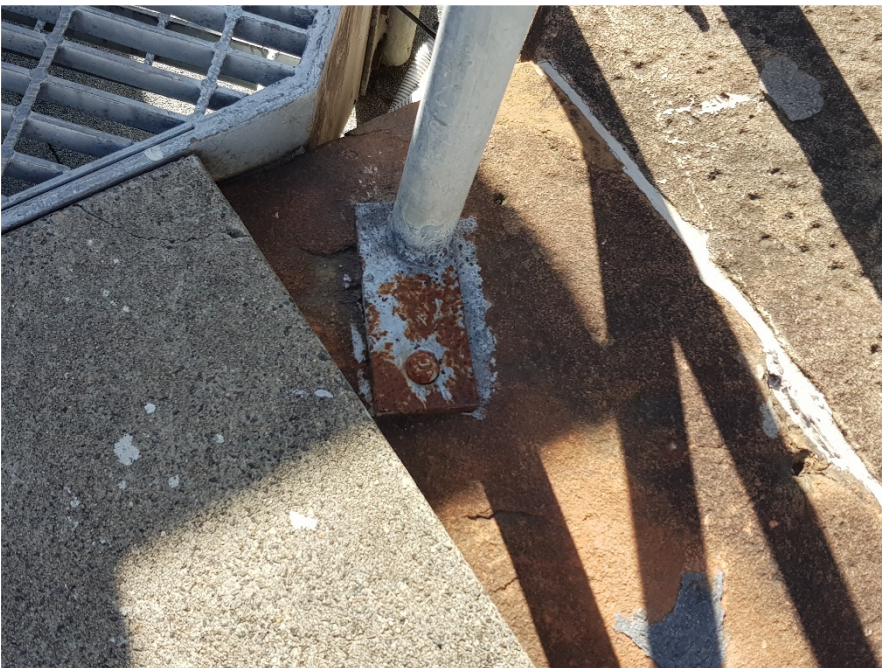
Figure 10: Corroded Connection of Access Structure South End
