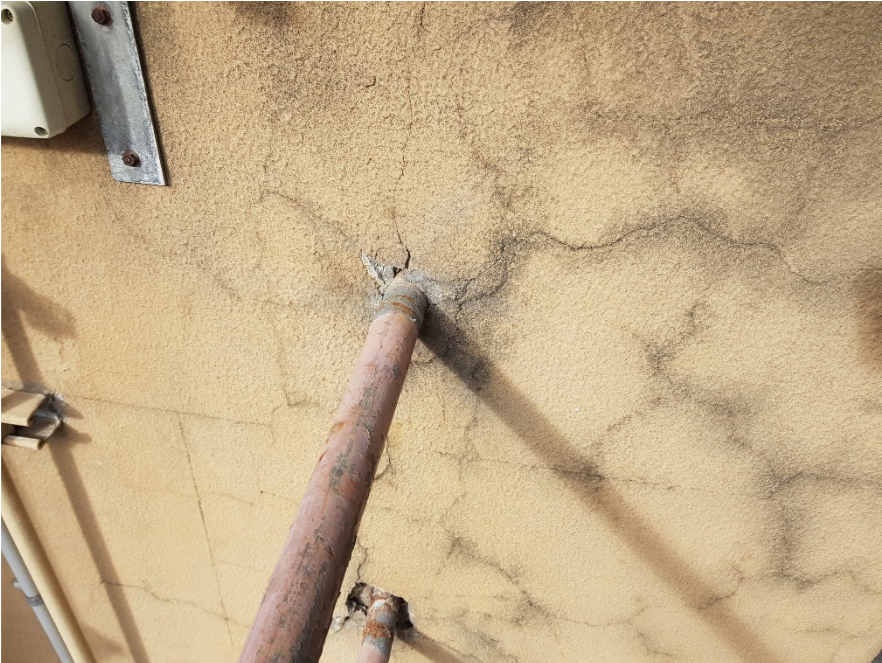
Figure 9: Cracking Around Embedded Railing
